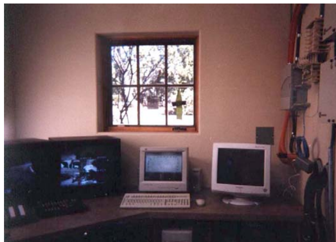
Fig. 2 - a typical observation post with the touch screen display for alarm annunciation (center) and a CCTV monitor (left).
